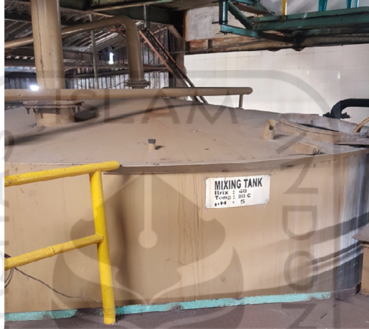
Gambar 4.1 Mixing Tank Pabrik Alkohol Jatiroto
