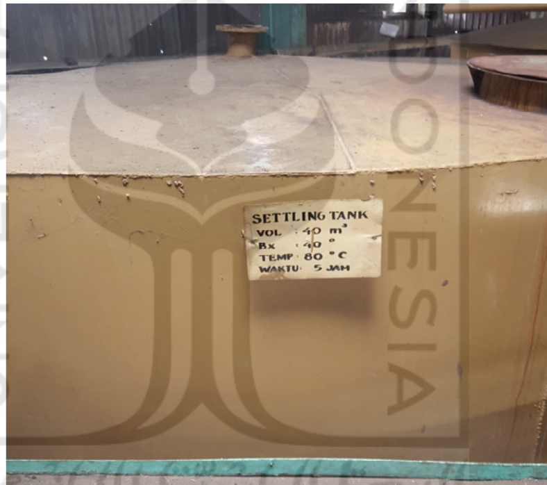
Gambar 4.2 Settling Tank Pabrik Alkohol Jatiroto
