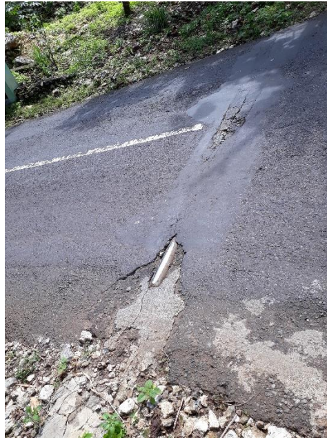
Gambar 1.5 Tambalan dan Galian Utilitas ( Patching and Utility Cuts )
