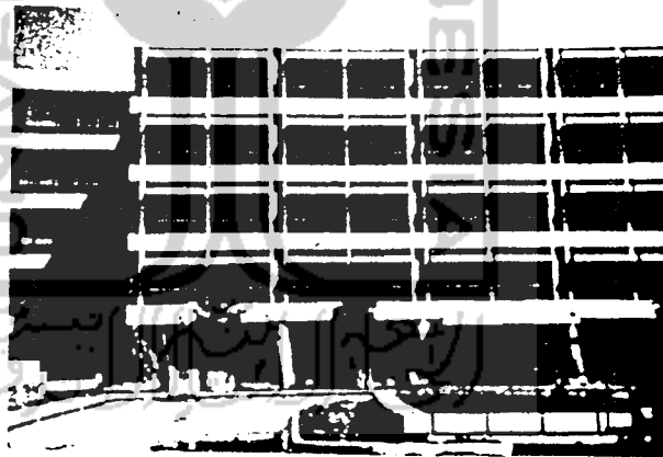
Gambar 2.5 Kerusakan akibat soft storey effects
