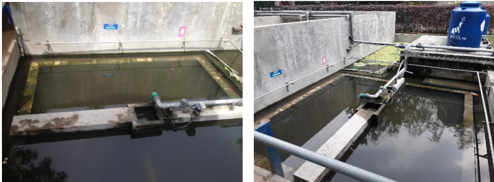
Gambar 4.16 Post Sedimentation Tank di unit IPAL Rumah Sakit “JIH” Yogyakarta
