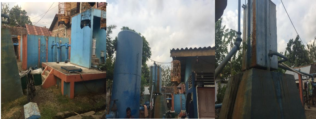
Instalasi Sewon PDAM Bantul Unit Sewon
