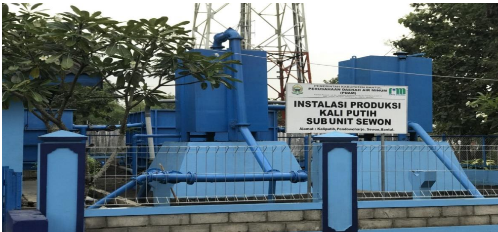
Instalasi Kaliputih PDAM Bantul Unit Sewon
