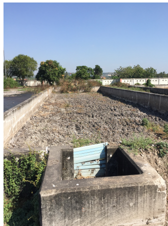
Gambar 4.14 Sludge Drying Bed
