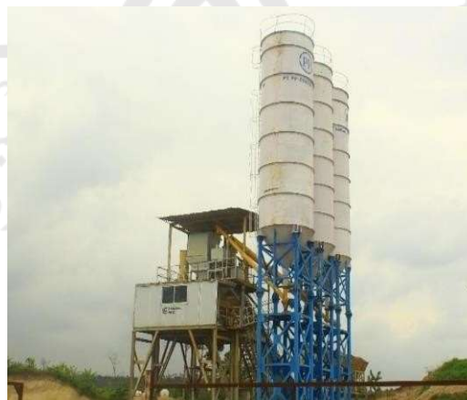
Gambar 25. Batching Plant Suplai Beton Kelas P
