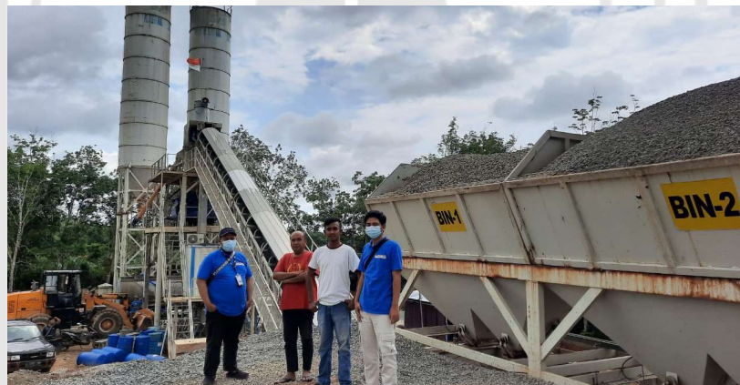
Gambar 80. Batching Plant PT. Semen Indogreen Sentosa
